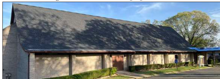
New roof on the Misión Creciendo en Cristo (Growing in Christ), North Little Rock church building (former Berean Baptist Church)
